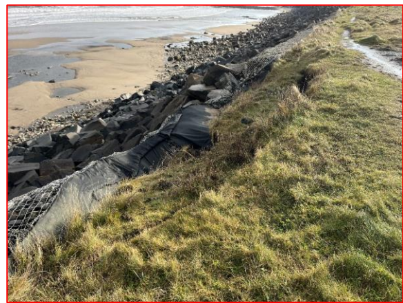
Localised cliff slide producing revetment movement and gabions failure on top of cliff (/4001C01)
