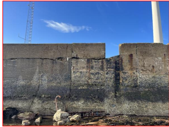
Corroded holdings and rotten timber screen – are in poor conditions and requires repairs (/4001C03)
