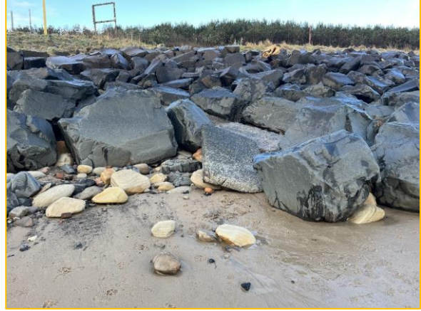
Displaced lower ramp from car park adjacent to redundant outfalls. (/3901C05)
