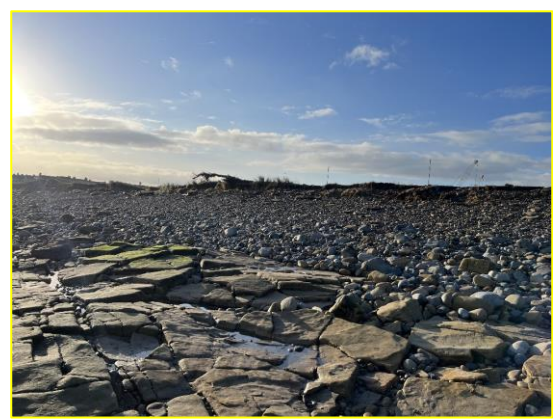
Accreted cobble berm flush with crest resulting in overtopping (/3901C04)
