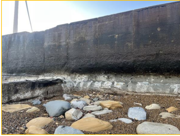
Severe undercutting of concrete wall to the north (/4001C04)
