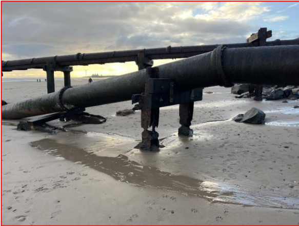
Low beach levels exposing further defects in abandoned outfalls (/3901C05)
