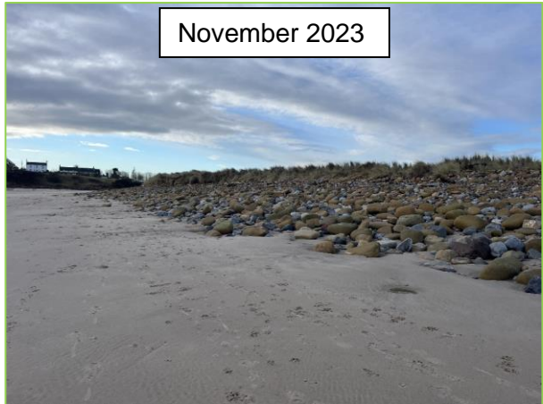
Lower beach levels at the same position post storms (/3801C01)
