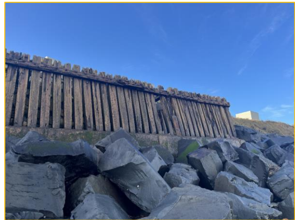
Corroded holdings and rotten timber screen – are in poor conditions and requires repairs (/4001C03)
