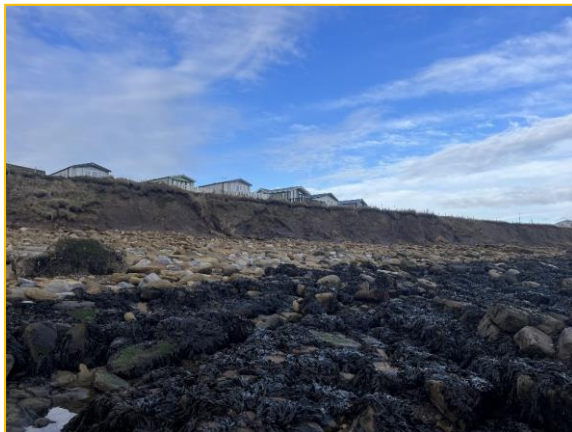
Eroding cliffs fronting Sandy Bay Caravan Park (/3701C03)
