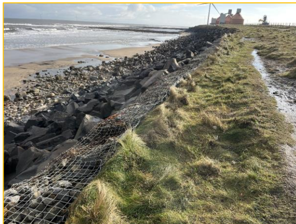
Rotated gabions adjacent to failed section (/4001C01)
