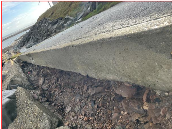
Ramp concrete slab undermining – needs to be repaired (/4001C01)
