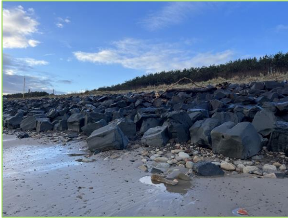
Rock revetment protecting former foundry site. Displaced lower rocks and storm debris visible (/3901C05)
