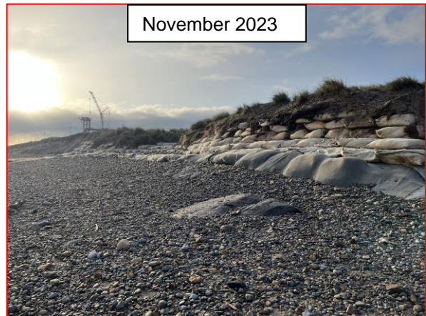
Exposed / damaged repair works (/3901C04)
