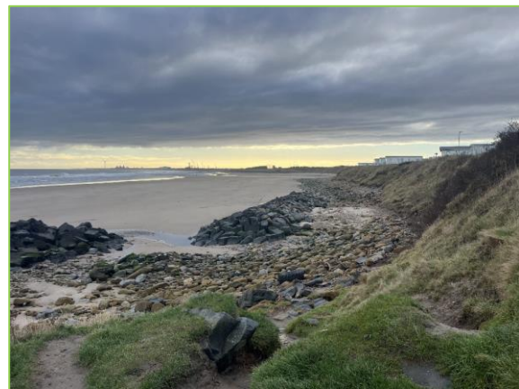
One of three near shore breakwaters offering protection to backing cliffs (/3701C03)
